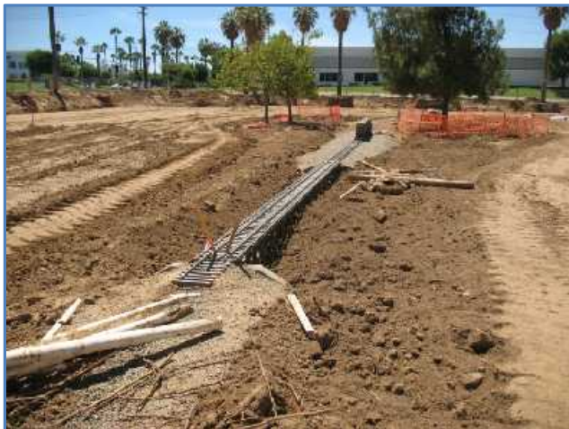
We were worried that we might lose our trestle. But the city and contractor assure us everything will be okay.
