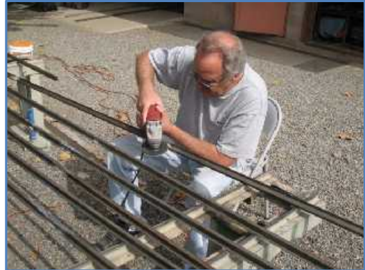
Using a grinder to smooth out the welds, Bob Smith prepares another length of steel rail for its placement along our mainline.
