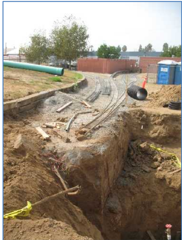
This trench tunneled under our compound lead and mainline then headed into Allen’s Valley. Fortunately, it’s completely buried now.
